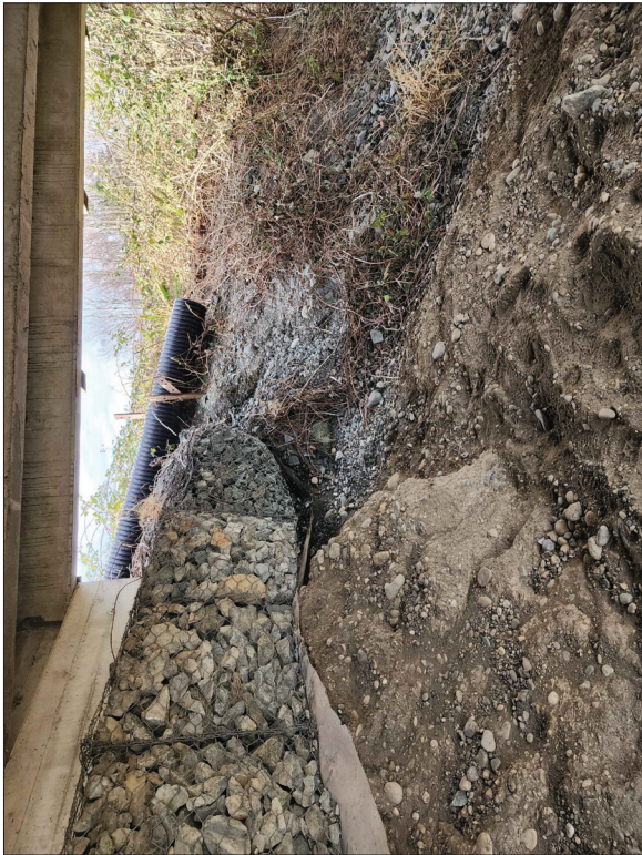
VIEW OF DAMAGED GABION FROM SOUTH ABUTMENT (LOOKING SOUTHEAST)
