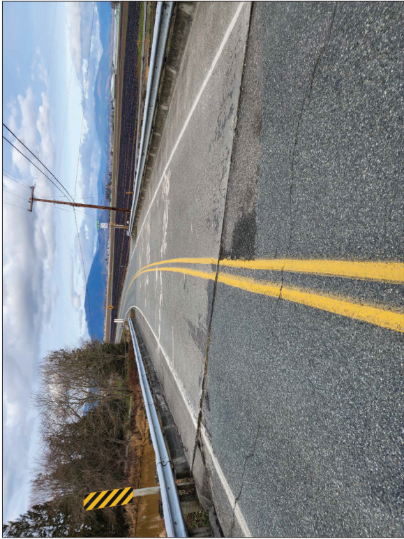
VIEW OF DAMAGED DECK AND SETTLING APPROACH ROADWAY FROM BAY VIEW-EDISON RD (LOOKING NORTH)
